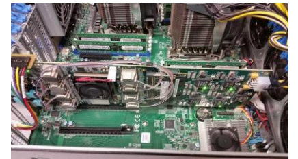
Installed in a PC
