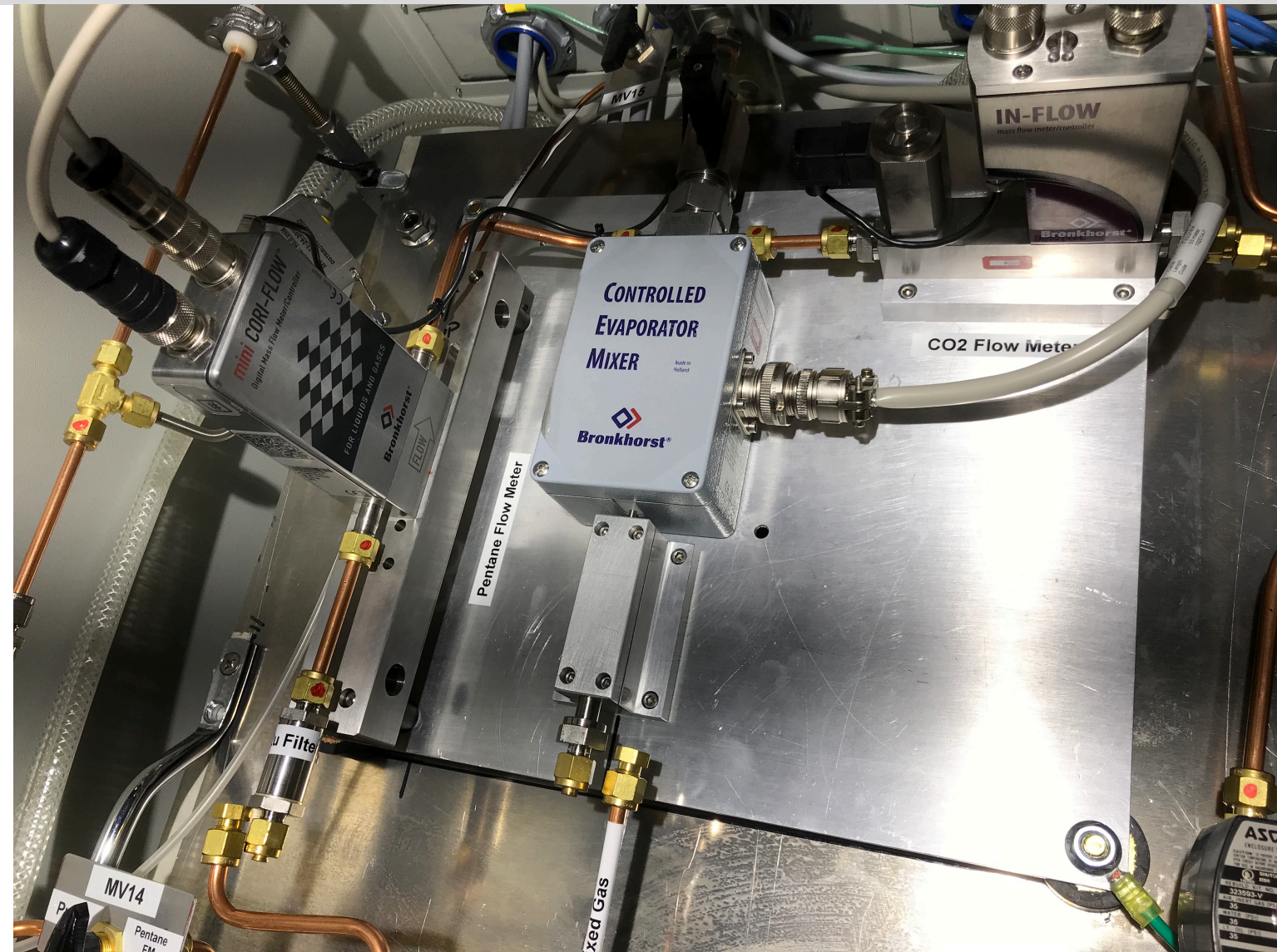
Bronkhorst components assembled in the gas cabinet
