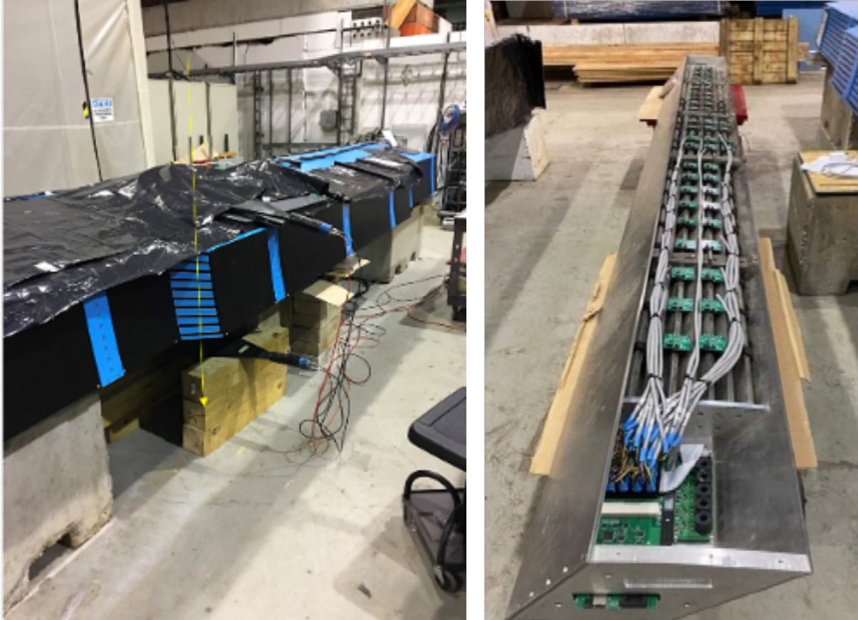
Figure 2.3: (left) Some of the outer HCal sectors being instrumented in Building 912 at BNL. All 32 sectors have been delivered and are awaiting the installation of scintillating tiles and electronics. (right) Inner HCal sector prototype. In the final design the iHCal structure is made of flat aluminum plates to minimize costs. The iHCal is also an important support structure for all the detectors inside the bore of the Babar superconducting solenoid.
