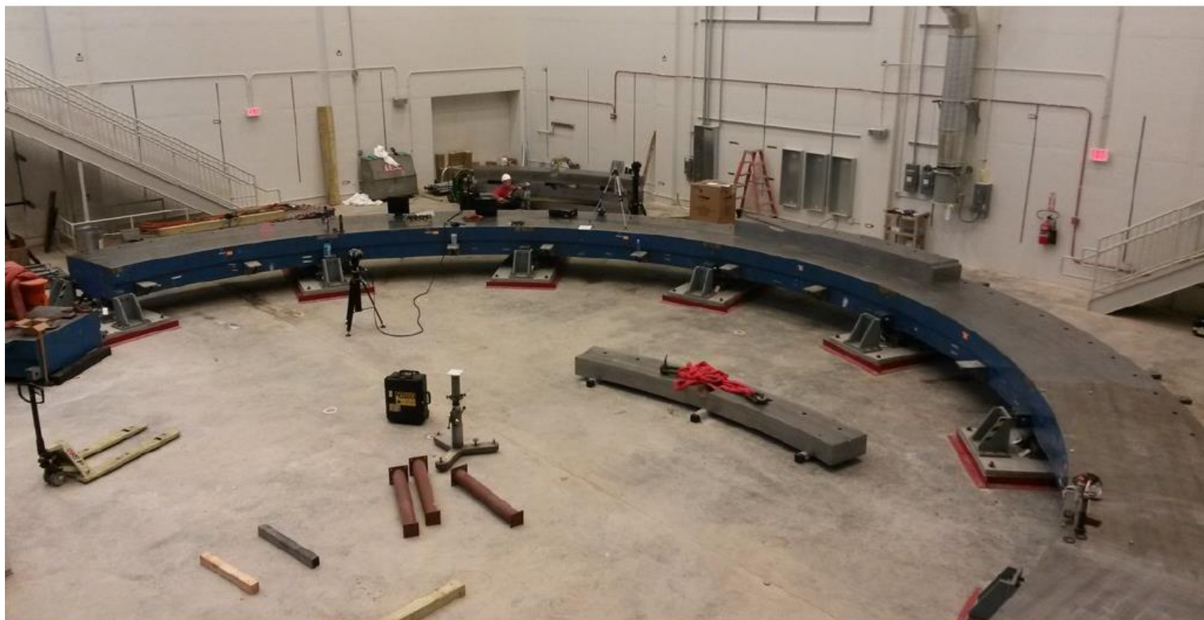
June 23, 2014. Bottom yoke. Reassembly progresses well. Superconducting coils will be moved into the experimental hall end of July 2014
