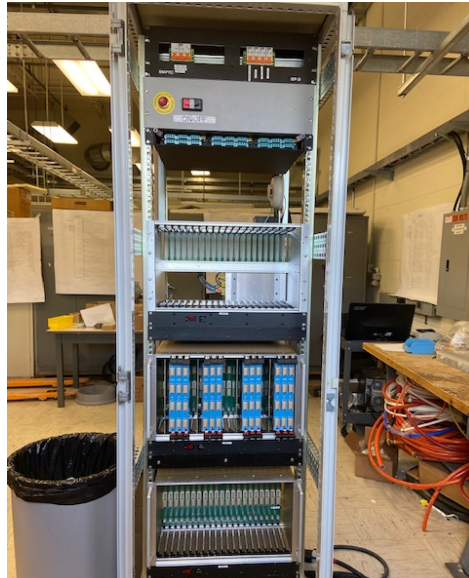
Figure 8: The first of 2 HCal Digitizer and Control racks being assembled in 1008. The racks will be installed on the second level of the detector and provide both slow control and readout of the HCal.
