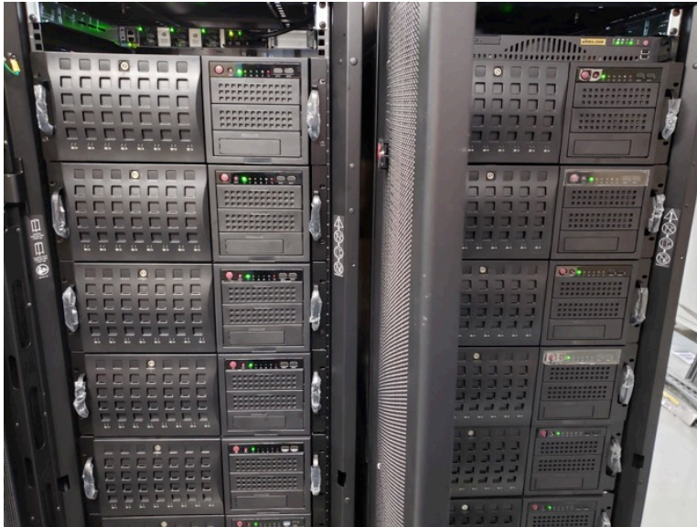
Figure 9: A picture of the two newly assembled racks with the new PCs.
