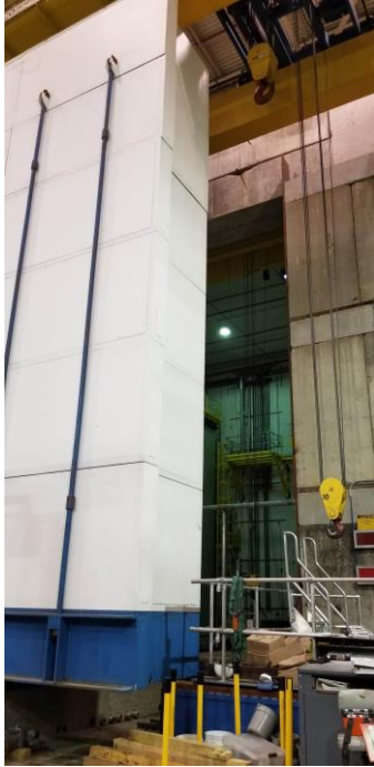
The shield wall pushed open
