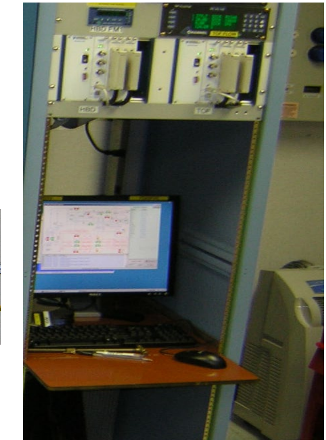
Existing TOF Controller and Flowmeters
