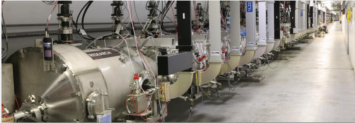
52-1/4 Cryomodules with 418 SRF Cavities to Accelerate Electrons in CEBAF
