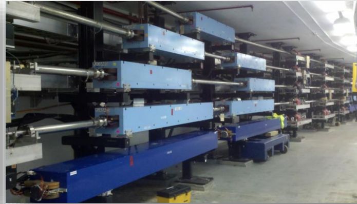
~500 Large Dipoles powered by >40 HVPS
