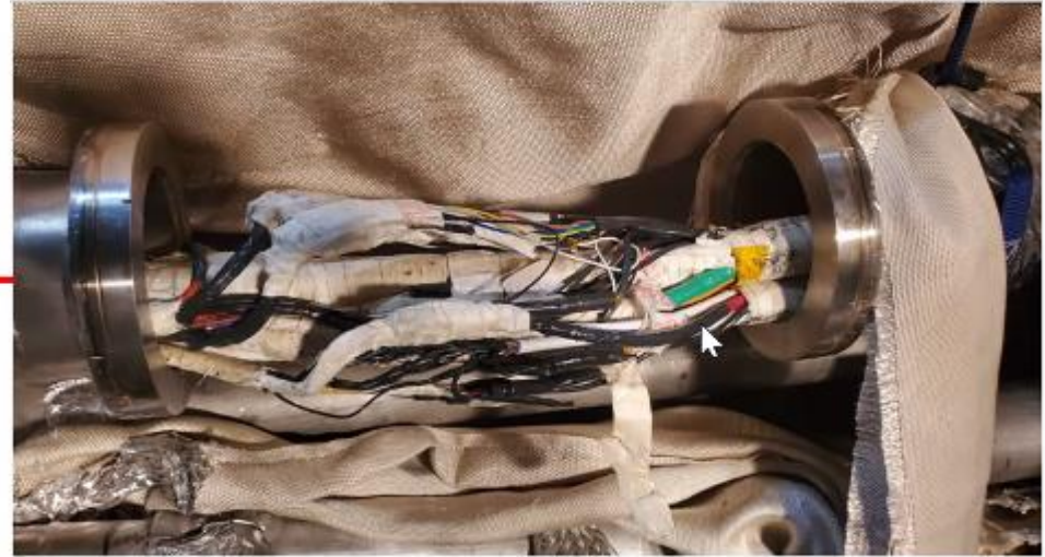
Splice can #1 (no trouble found)
