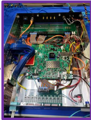
Global Timing Module (NSLS II/sPHENIX) Receiving from RHIC RF low jitter clock source
