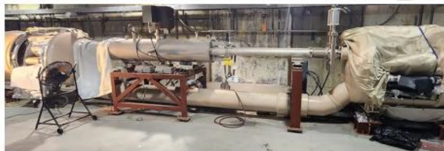
Inside the RHIC tunnel
