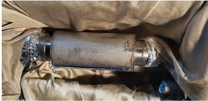
Splice can (#1) before opening
