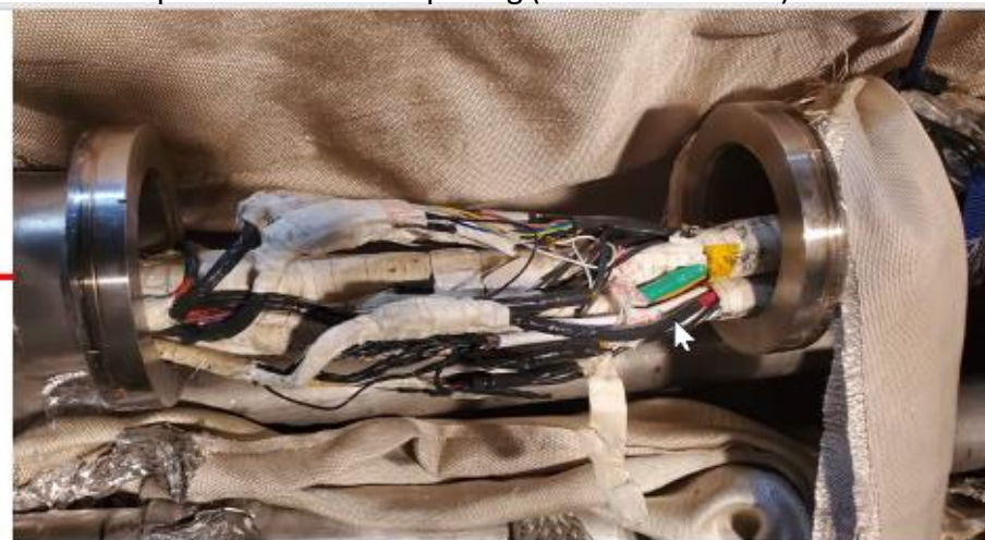
splice can #1 after opening (no trouble found)
