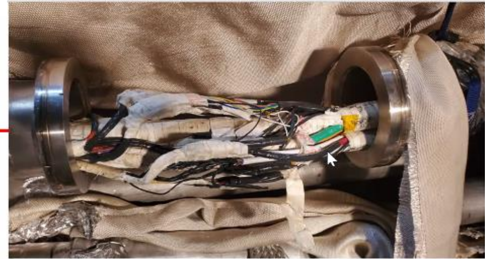
Splice can #1 after opening (no trouble found)
