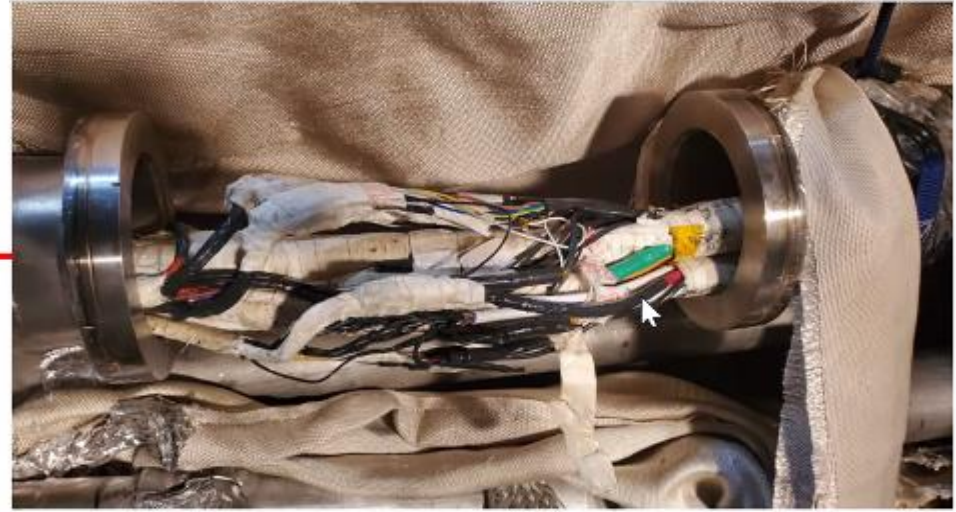
Splice can #1 after opening (no trouble found)
