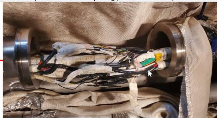
splice can #1 after opening (no trouble found)
