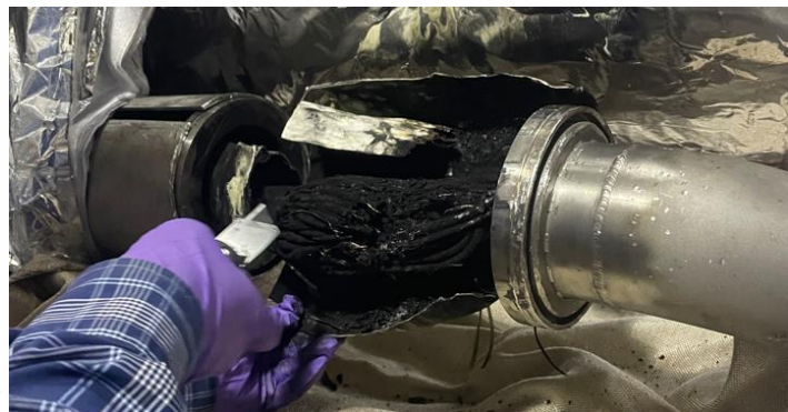
damage inside splice can
