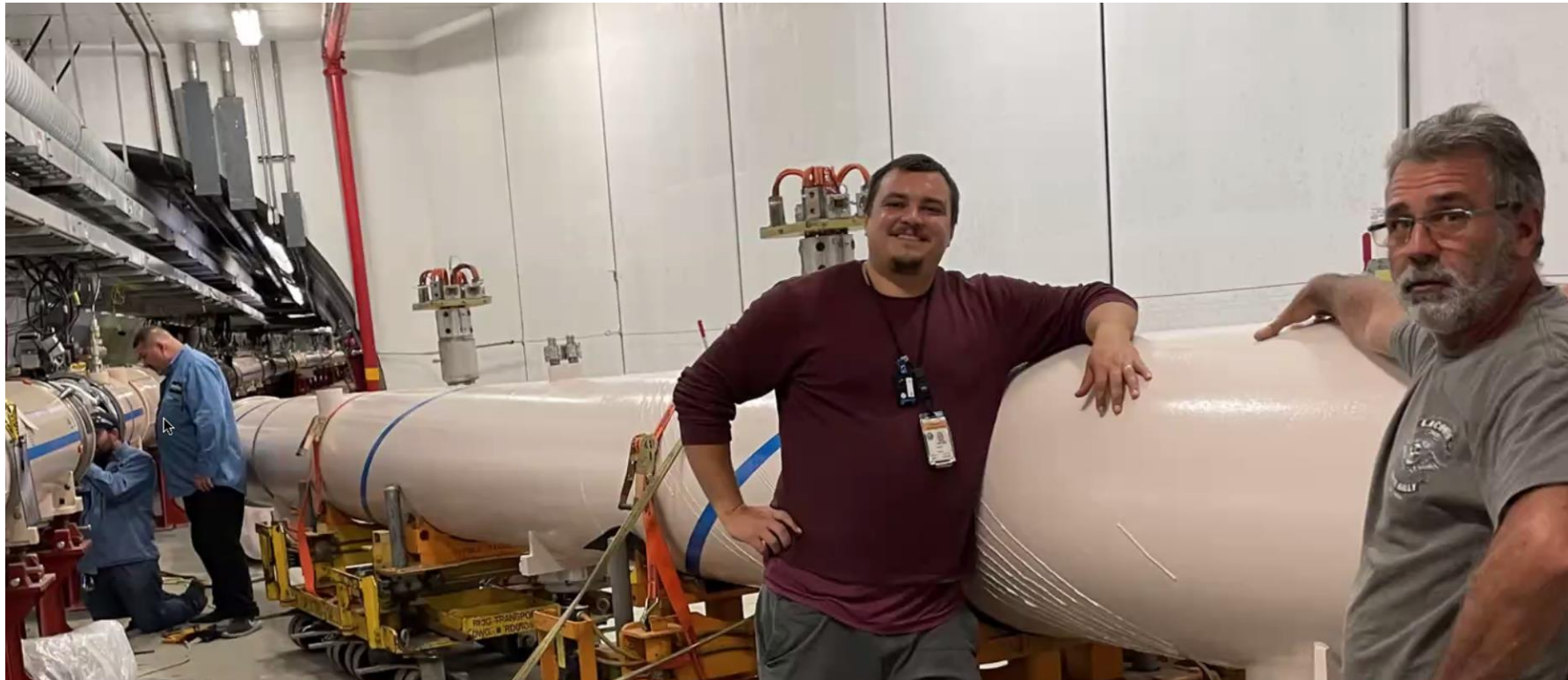
Dummy magnet and snake in RHIC tunnel prior to removal/installation/survey (IR8 region)
