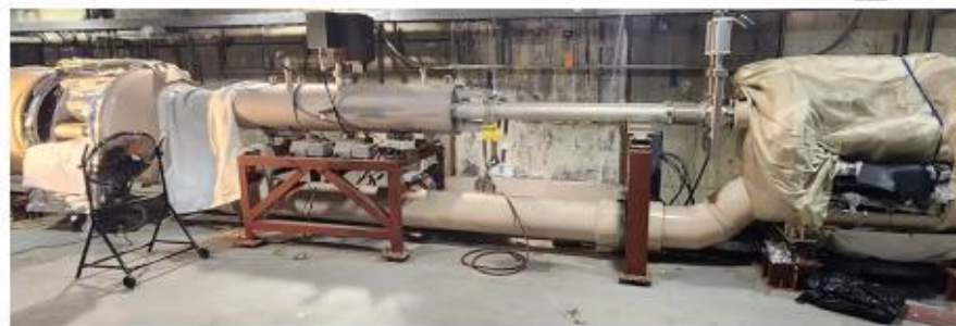
Inside the RHIC tunnel
