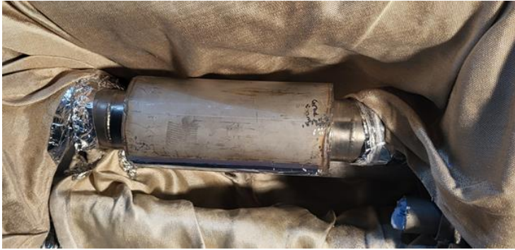
Splice can (#1) before opening
