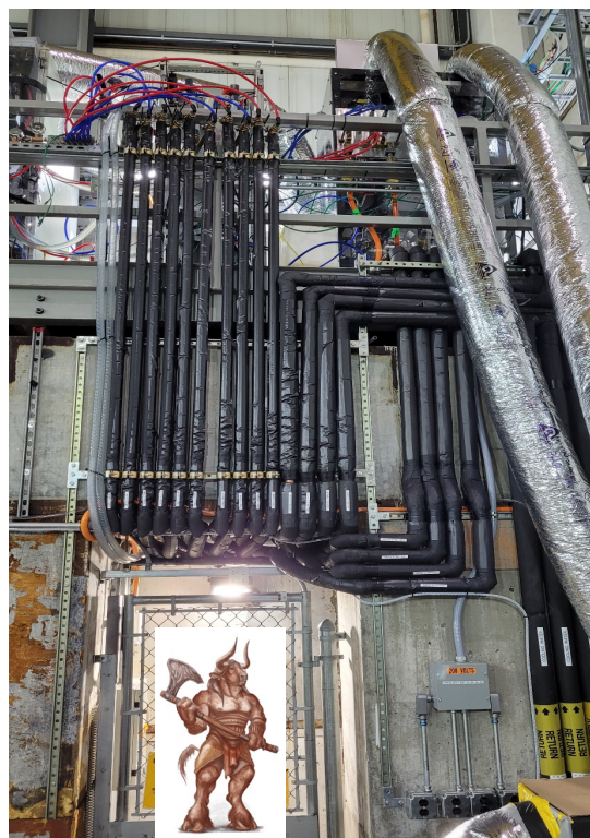
MVTX Longer Term Solution running additional lines through labyrinth (from chiller platform into IR)
