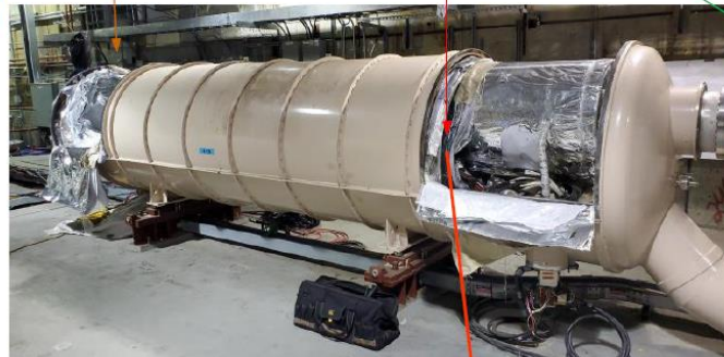
Splice can #3 is removed after found the arcing at splice.
