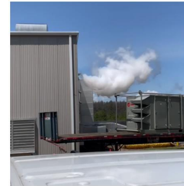
Helium venting at Bldg. 1004B
