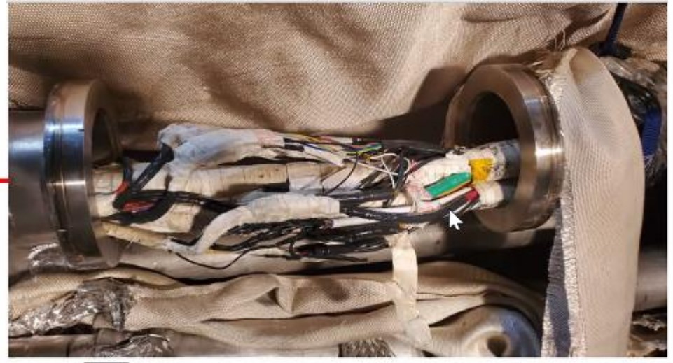
Splice can #1 after opening (no trouble found)
