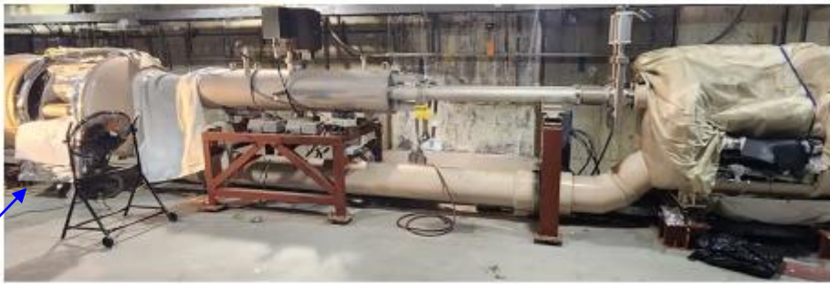
Inside the RHIC tunnel
