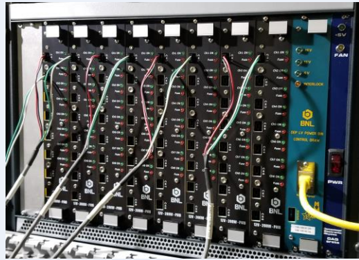
Turned DEP crates into Custom 2kW LV power bin x2
