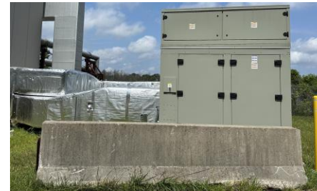
1004B Replacement AC
