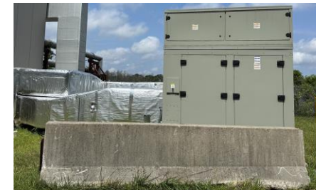
1004B Replacement AC
