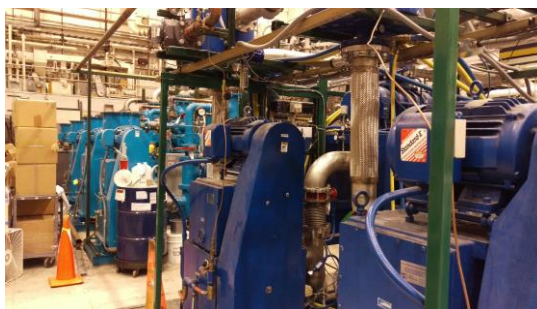
Blower Pumps (4 m away) No direct contribution
