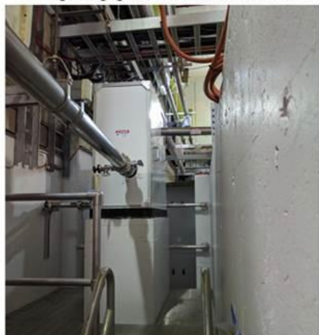
Relay table enclosure with laser transport pipes to LEReC and CeC
