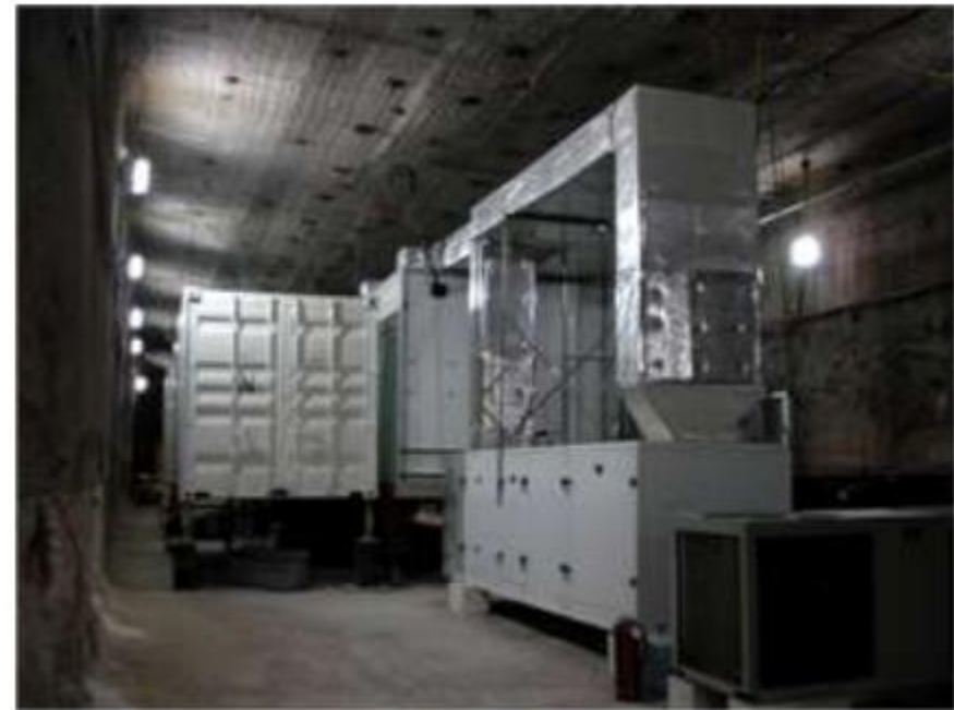
Cleanrooms at WIPP drift
