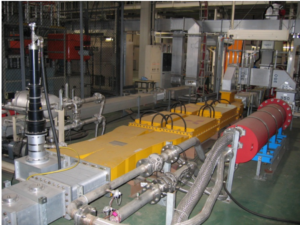
RF high power system
